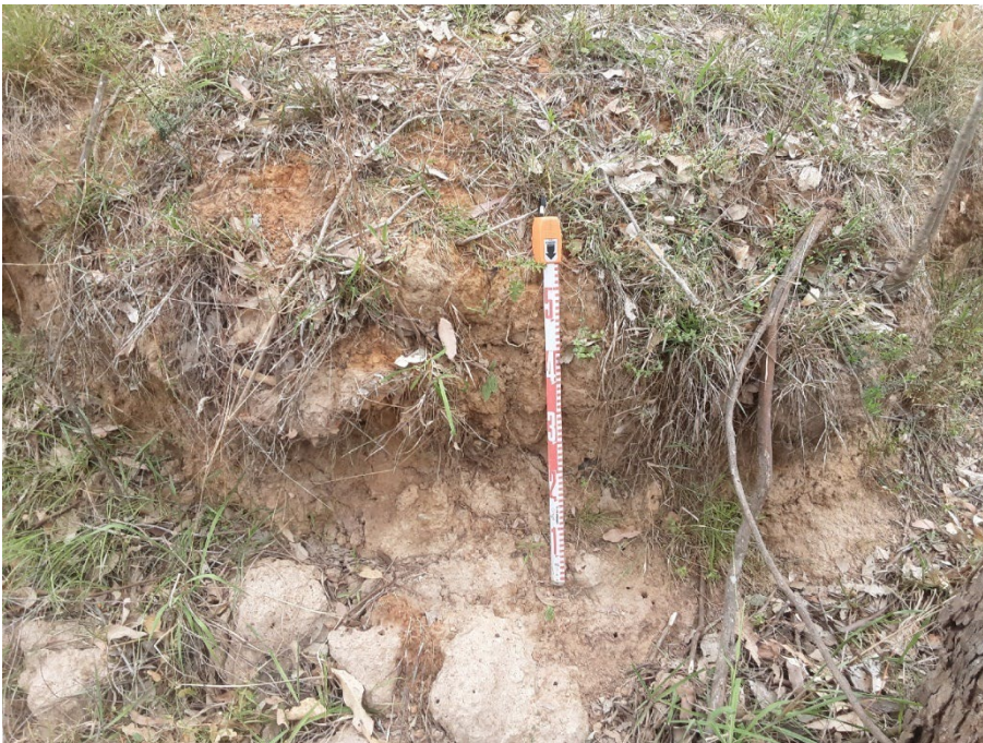
Photo 15 Area of exposure on eroded wall of drainage line (0.5 metre scale)
